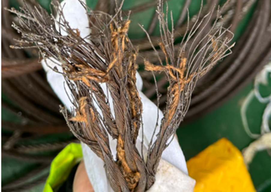
Figure 21: Wire rope breakage.
